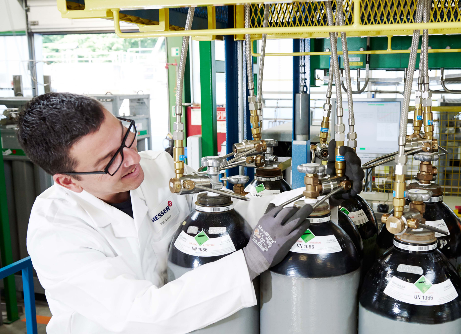
Filling station for high-purity gases
